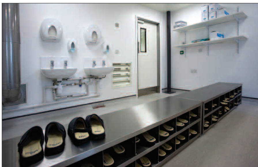
A stainless steel bench, running across each gowning room, maintains a barrier between external and process areas.
