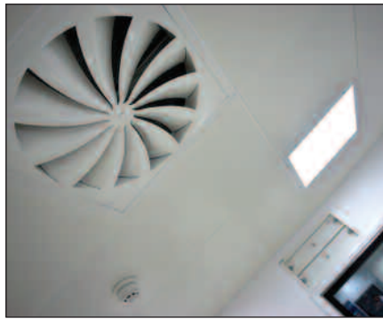
A supply air diffuser in the centre's metal pan ceiling, with a viewing window and pressure stabiliser to the rear.
