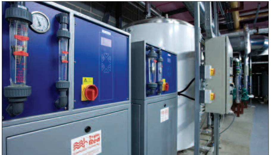
The Triple Red reverse osmosis equipment used to purify mains water.
